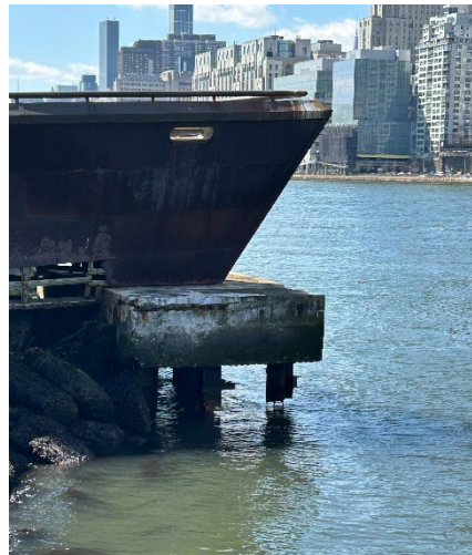
Overview of north side of pier showing deterioration of Corten panels and of mooring pad.
